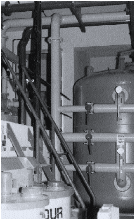
A view of one of the many filters, pipes and equipment placed to recycle water.
